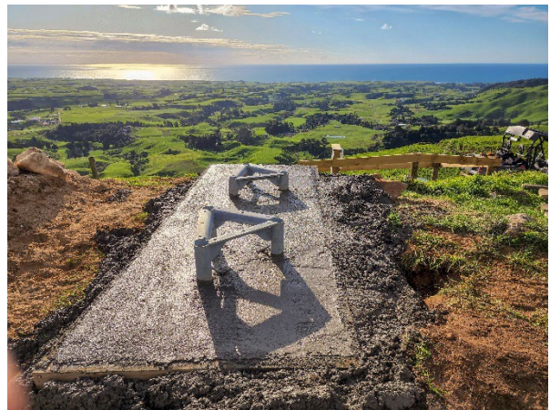
Concrete base pad down and ready to be cleaned up for the above-ground sections of the tower.
