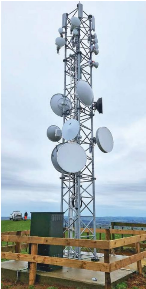
Tapp Road tower, Lightwire, Rural Capacity Upgrade Programme
